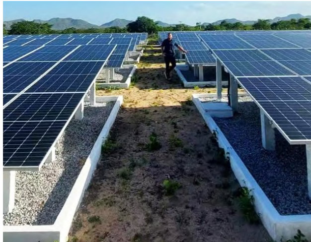
1.5 MW Ground-mounted PV Plant 3260 pcs mono half-cut 460W
