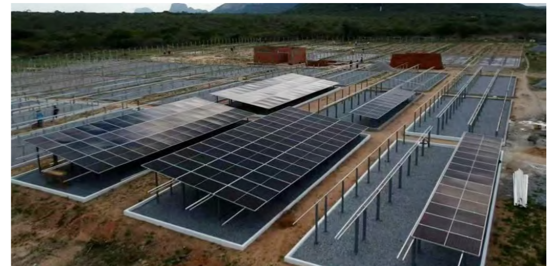
1.3MW Ground-mounted PV Plant 2364 pcs mono half-cut 550W
