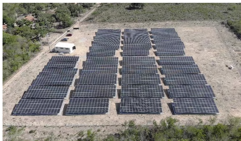
2.8MW Ground-mounted PV Plant 6222 pcs mono half-cut 450W
