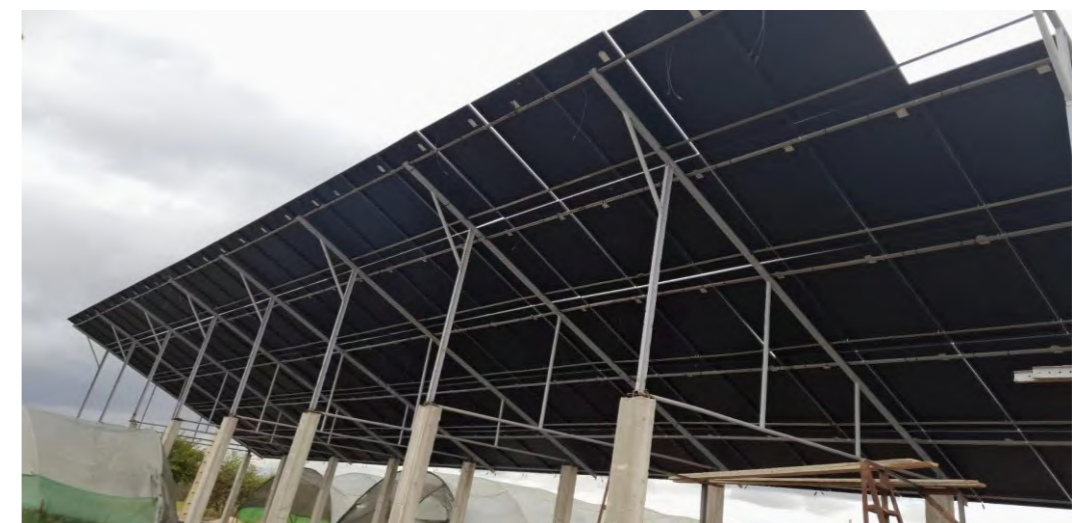
55KW Ground-mounted PV Plant 100 pcs mono half-cut 550W
