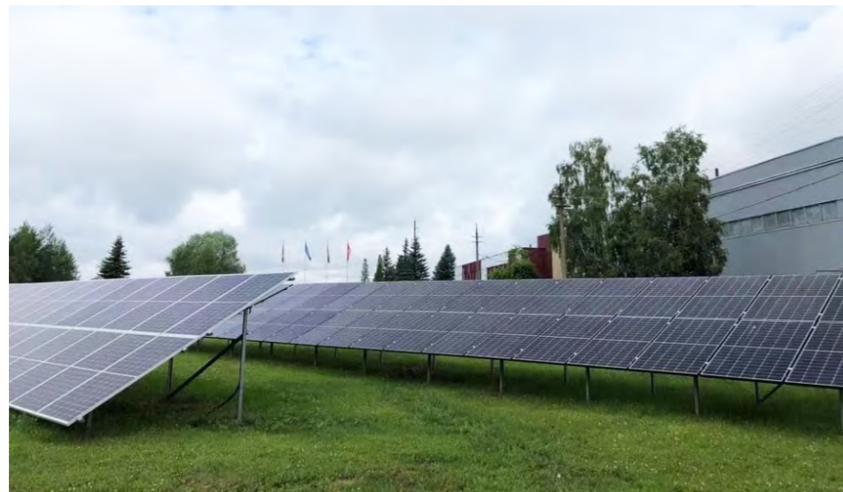
80KW Ground-mounted PV Plant 216 pcs mono half-cut 460W
