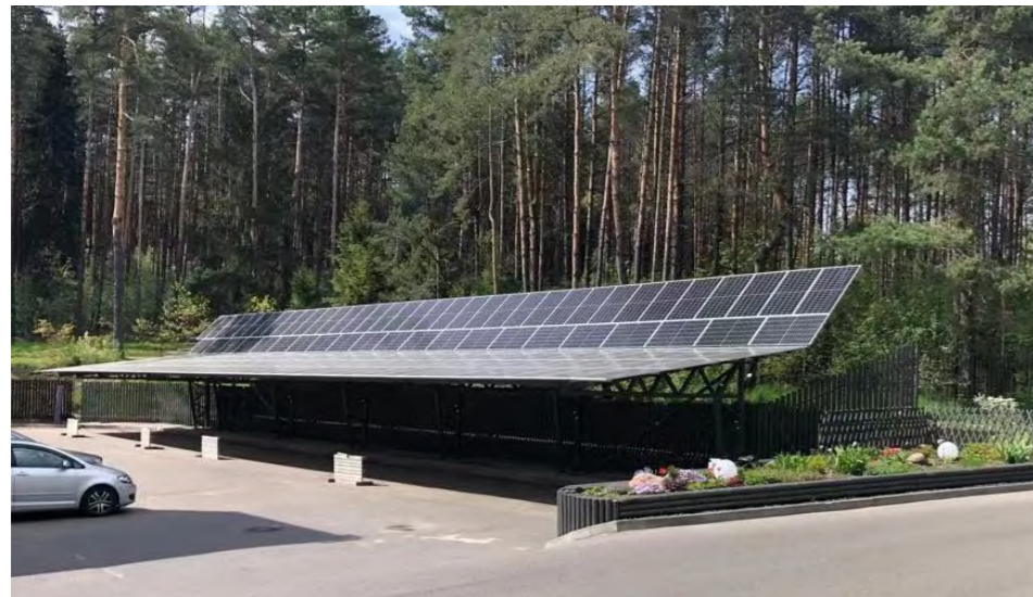
65KW Carport PV Plant 176 pcs mono half-cut 370W
