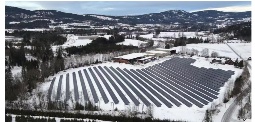
6MW Ground-mounted PV Plant 3260 pcs mono half-cut 460W
